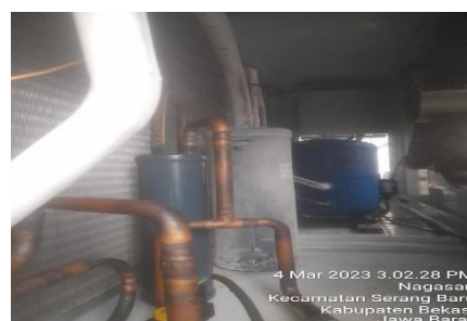
Figure 6. Freezing on gas lines
